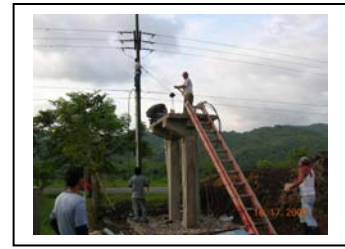
Installing transformer onto elevated platform from which all wires will then run underground to clinic
